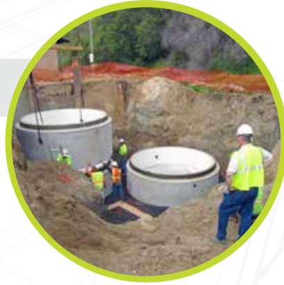
Water & Sewage System Waste Treatment Facilities
